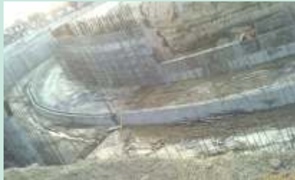
Project: Rail underpass • Location: Sanjay Gandhi Transport Nagar, Delhi • Client: Railway • Status: In progress
